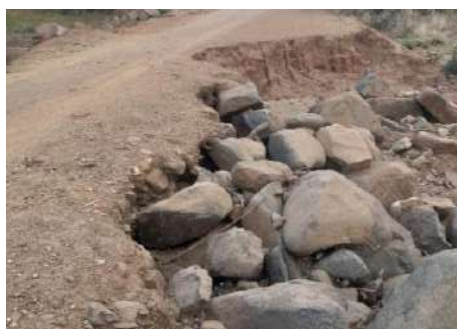
Part of Damaged Road right side
