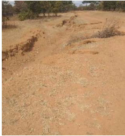
Part of Damaged Road Section
