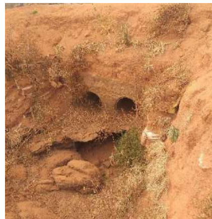
Old Culverts Not Replaced
